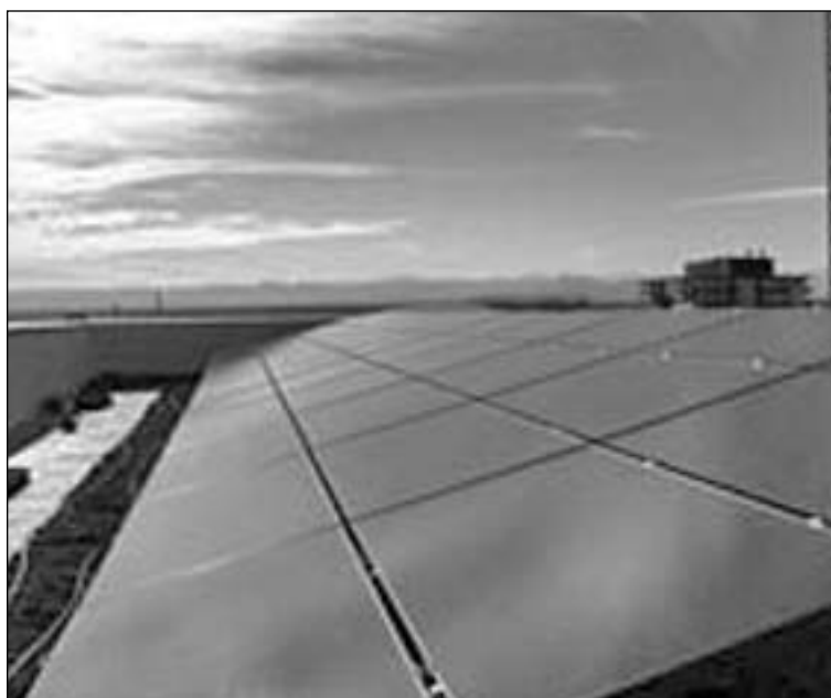
SOLAR PANELS WHICH ADORN THE DENVER OFFICE OF THE EPA. PHOTO COURTESY OF EPA.GOV
