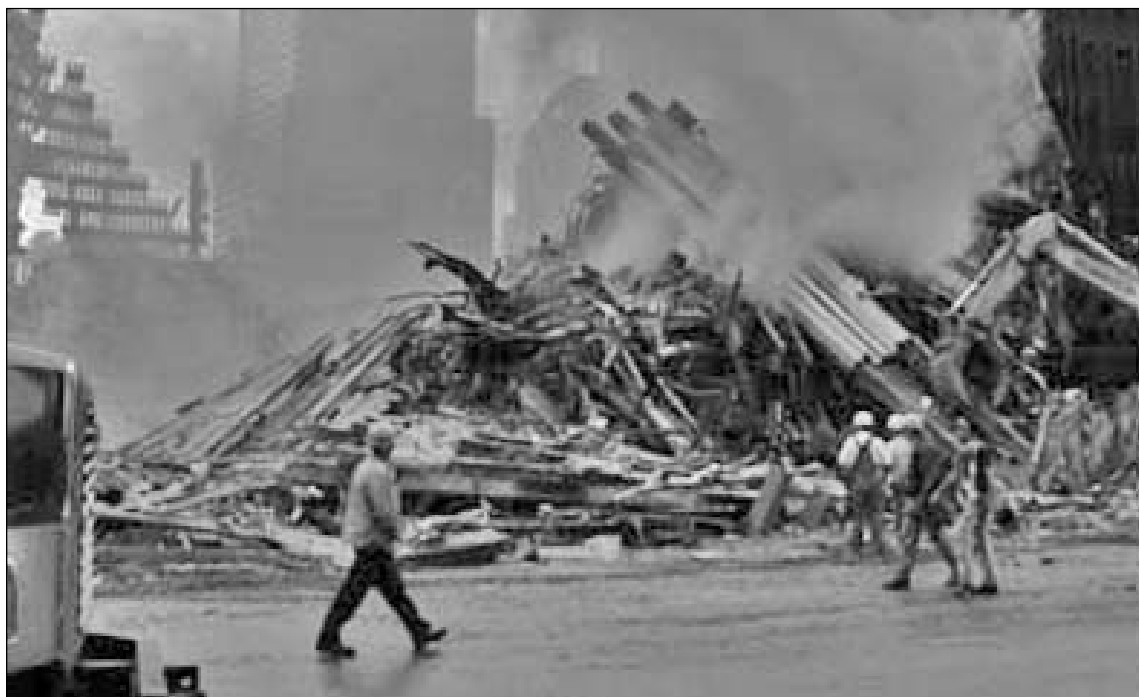
Rescue workers help clear away the rubble at ground zero. Photo provided by www.epa.gov
